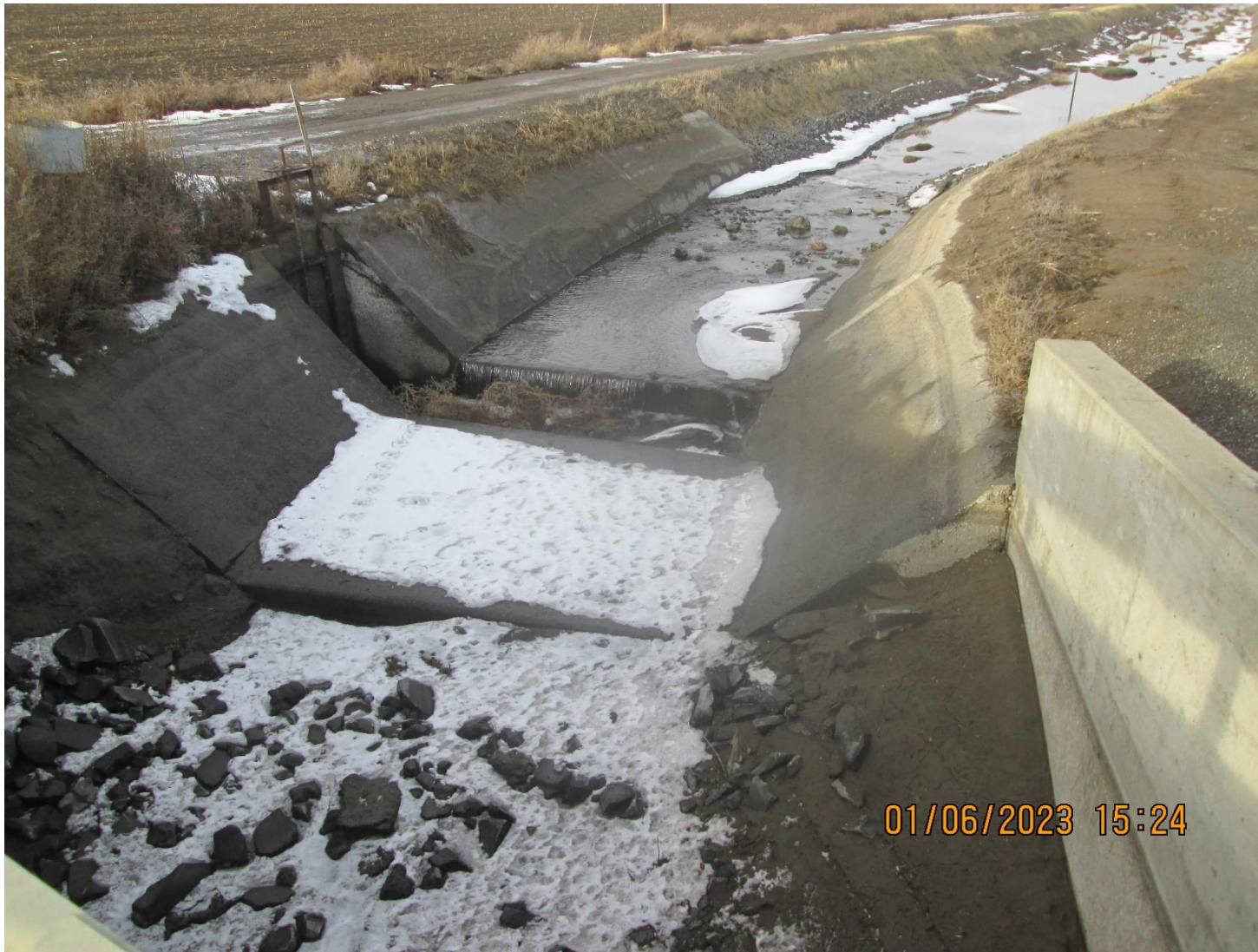
North South Drain next to Nichols Road – Drains into the Granger Drain
