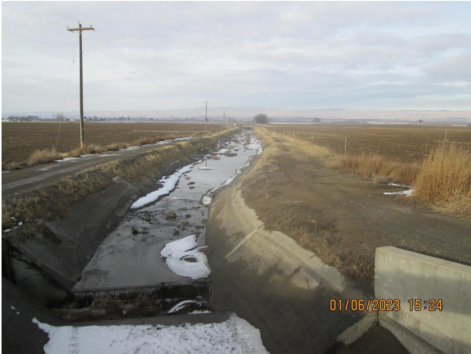
North South Drain next to Nichols Road – Drains into the Granger Drain
